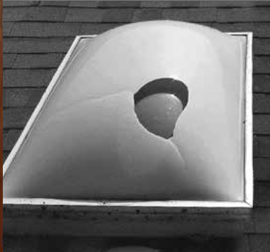
Old acrylic domes can be easily damaged.
